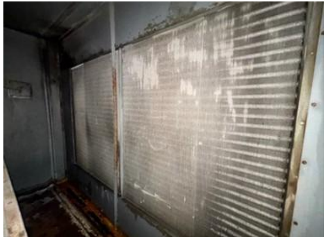
After cleaning, grooves and fins are visible.
