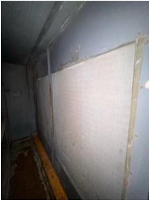
Dirty coils before cleaning.
