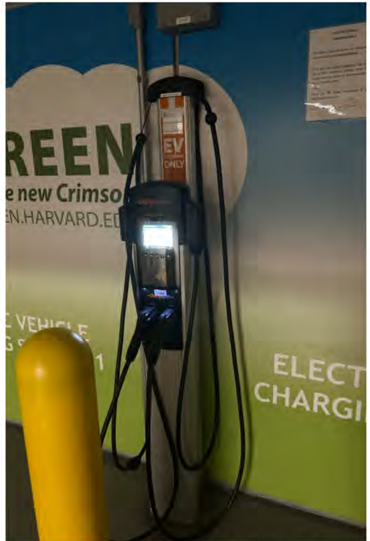
ChargePoint EV Charger in VSC Parking Garage
