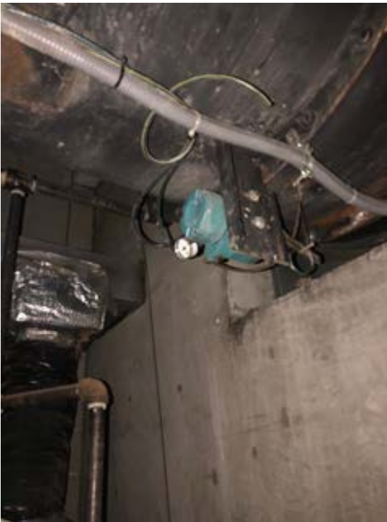
Guide vane, controls the speed of the fan.
