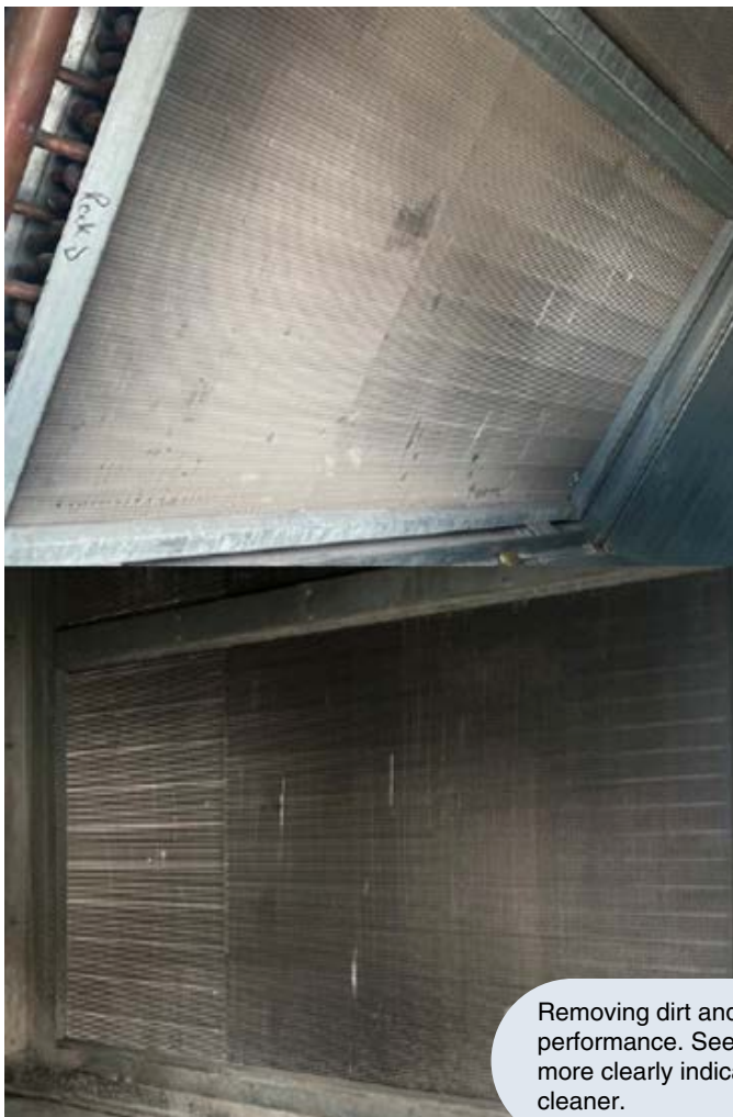
Coils before cleaning
