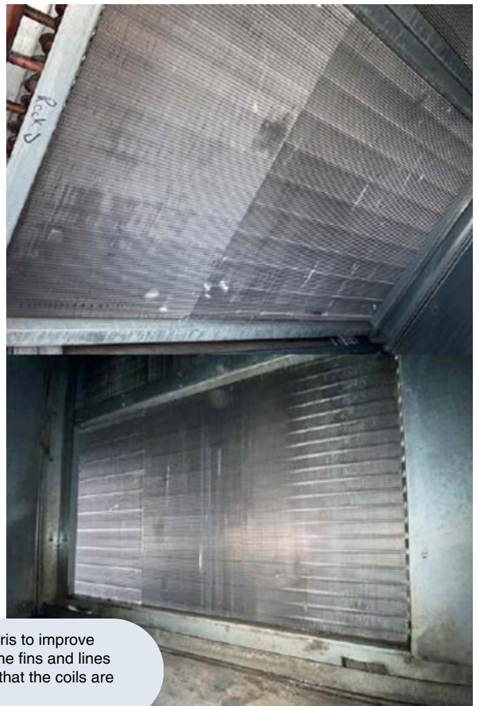
Coils after cleaning
