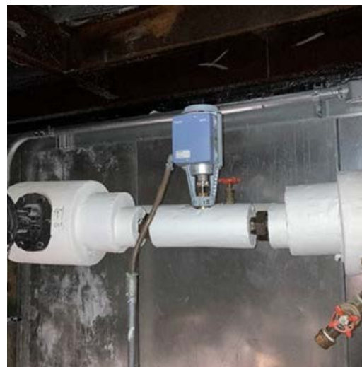
New steam control valve on air handling unit
